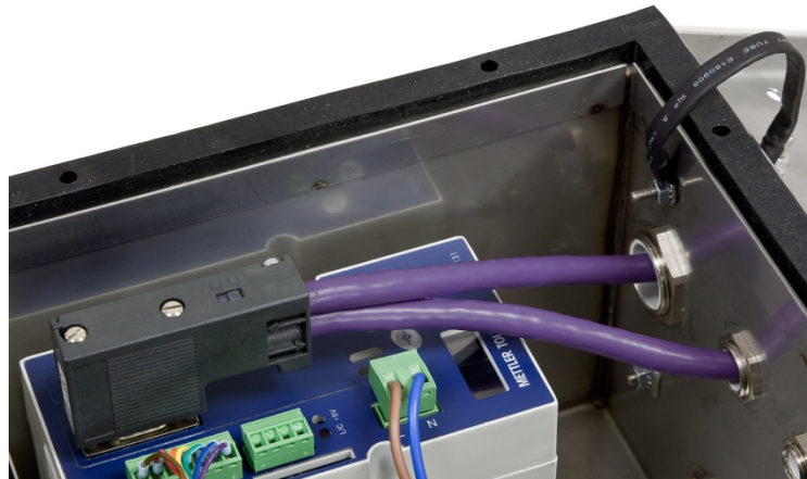
Figure 2-71: Updated J-Box Enclosure PROFIBUS Cable Routing
