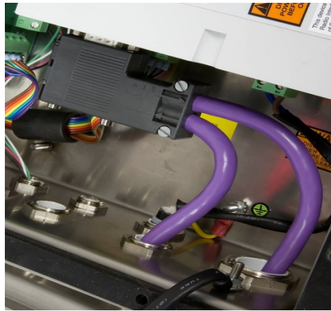
Figure 2-70: Original J-Box Enclosure PROFIBUS Cable Routing
